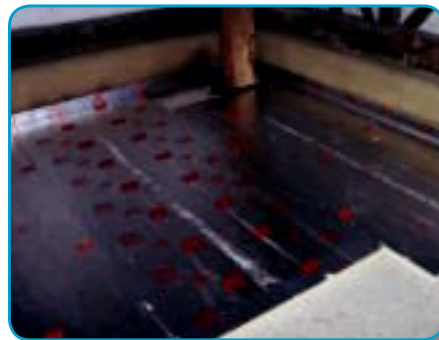
The floor is cleared of dust and debris and insulation is laid across the area.
