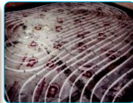
Speedfit pipe is laid in a pre-determined pattern and fixed in position with staples.
